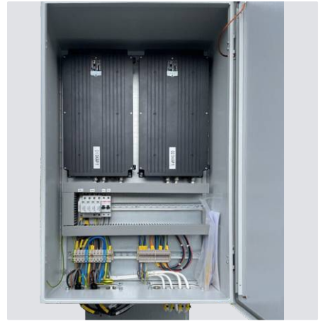
Control Gear put in the electric cabinet
