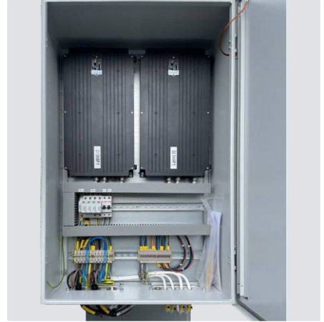
Control Gear put in the electric cabinet
