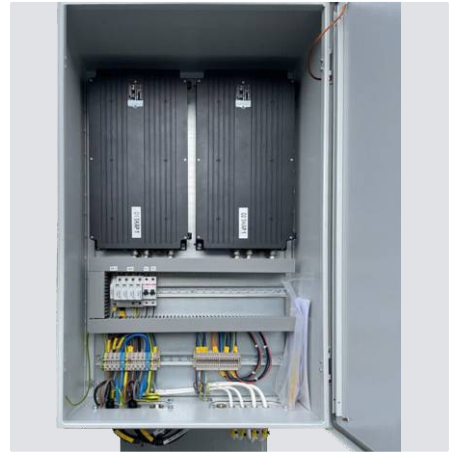
Control Gear put in the electric cabinet
