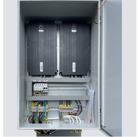
Control Gear put in the electric cabinet
