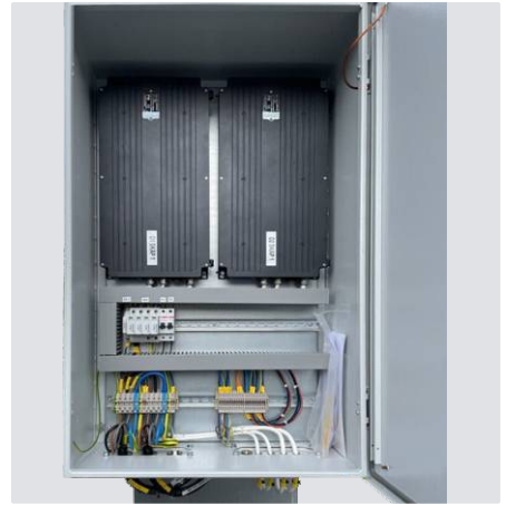
Control Gear put in the electric cabinet
