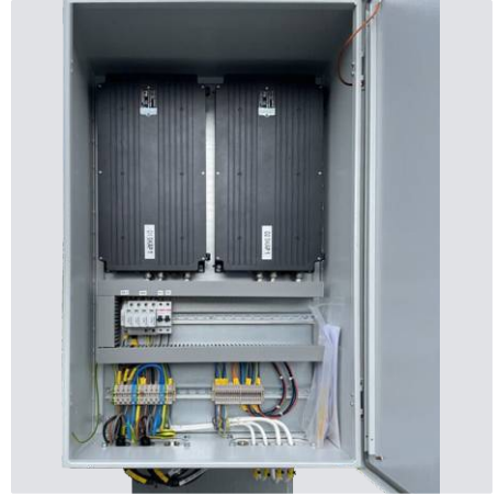
Control Gear put in the electric cabinet
