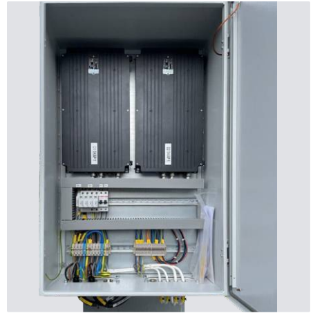
Control Gear put in the electric cabinet
