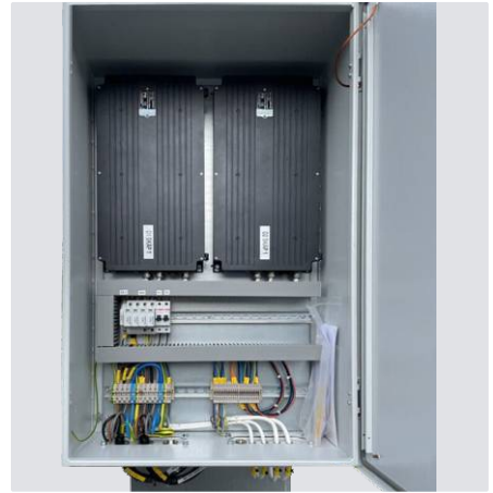
Control Gear put in the electric cabinet
